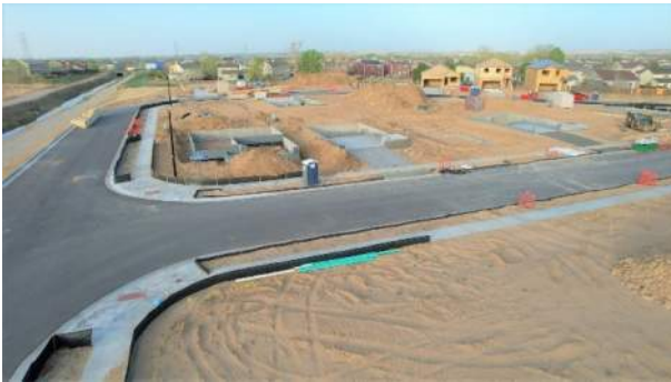
Foundations and Vertical Construction moving forward at the corner of Sunrise Drive and Ledge Street
